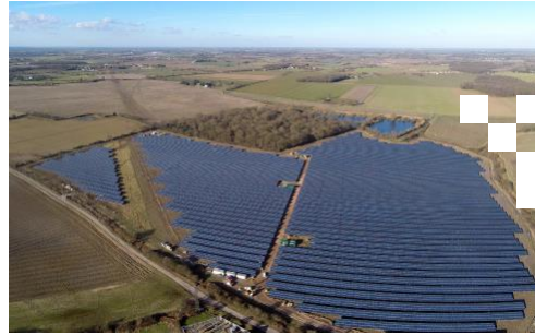
PV Utility-Scale Chisbon (UK)
